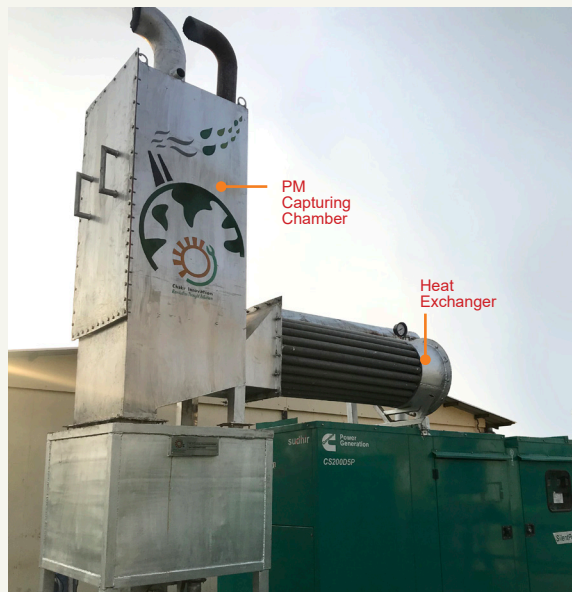
Chakr Shield retrofitted on a DG set
