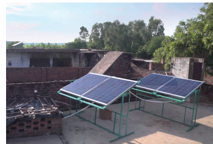
Boond's microgrid installed at Para Village, Uttar Pradesh
